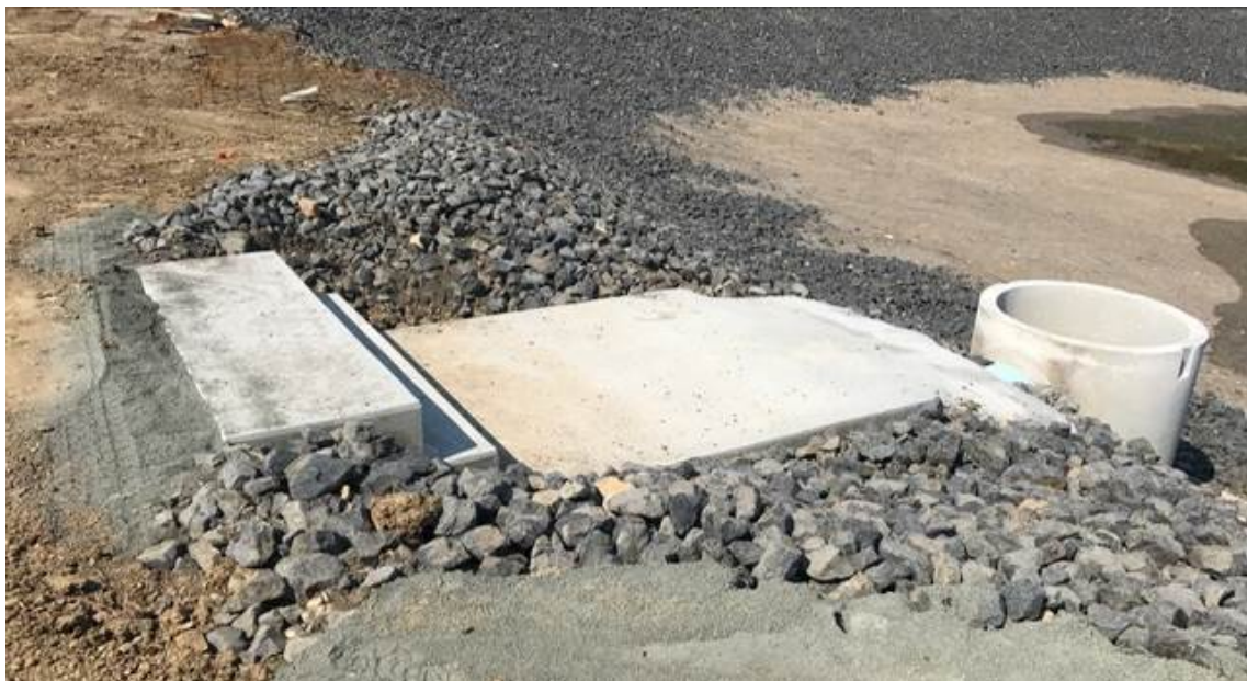
Figure 9.8.1 - Storage Pond Outlet Interior
