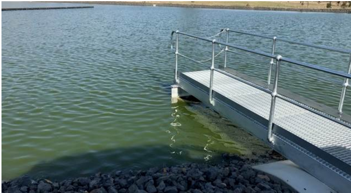
Figure 9.8.3 - Maturation Pond at Capacity
