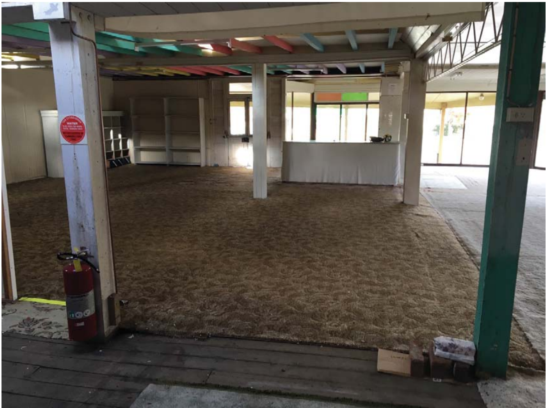
38W Fitzroy Street - Crafts Store, internal view towards Fitzroy Street (Image: Studio Two Architecture 26/06/2019)
