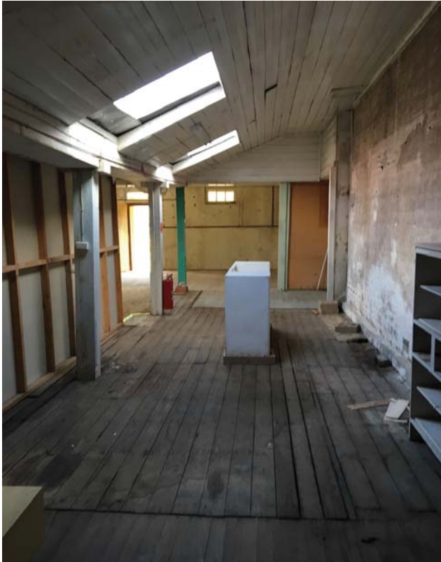
View of 38W Fitzroy Street - Crafts Store, internal view (Image: Studio Two Architecture 26/06/2019)
